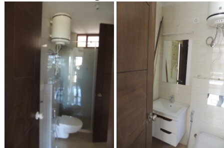
Fully Equipped Toilet with Shower Cabin Geyser, fitting & Fixture.
